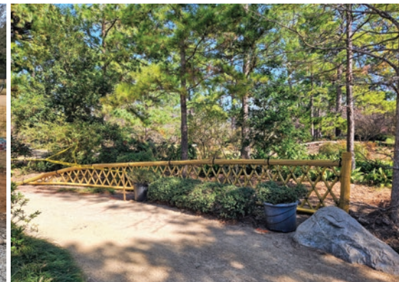
Another project completed during the two-week visit was the installation of a new screening "Koetsujini" fence adjacent to the Tea House.
